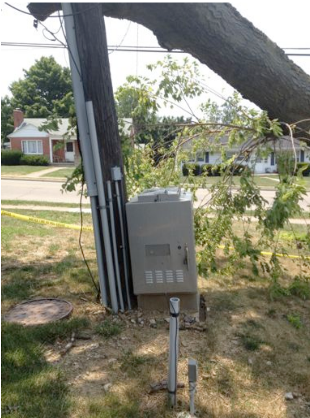
a view of the utility pole and our radio cabinet. The cabinet was, essentially, untouched; however it is securely bolted to the pole.
