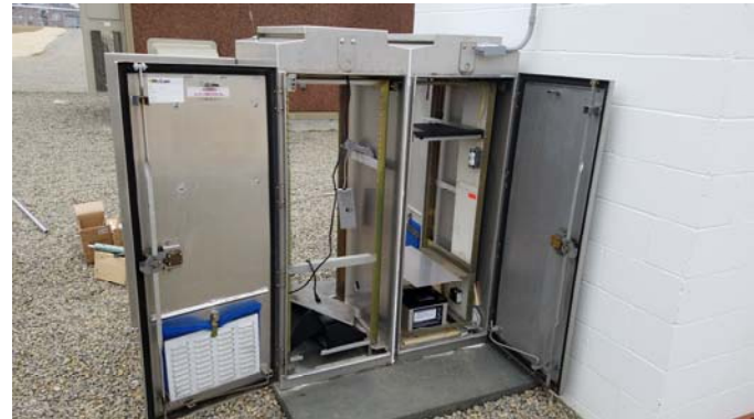
Empty repeater cabinets with batteries in place
